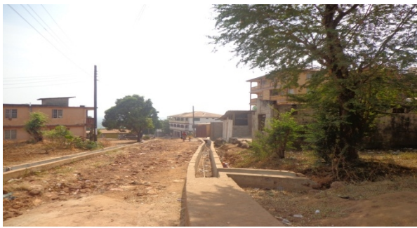
Construction of Side drains and Vehicular Slab at Cemetery Road, Lower Allen Town
